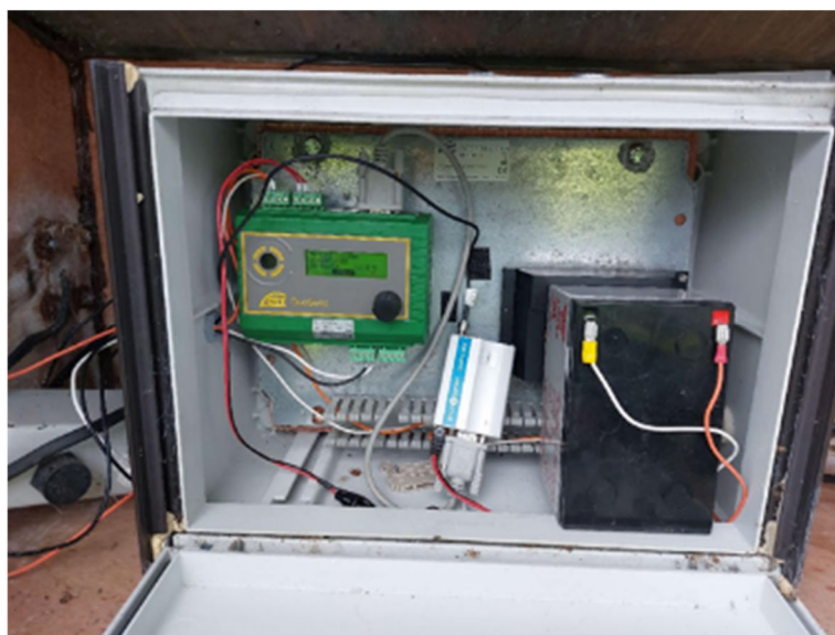
Figure 2-3: Aggard Bridge 29010 Data Logger
