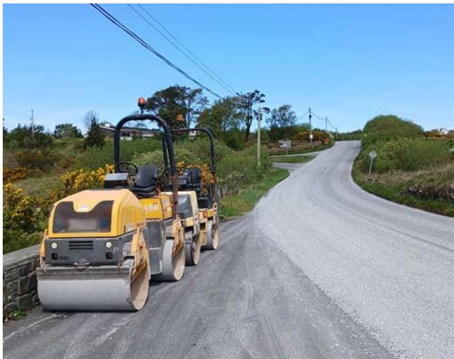
CS-RM-01 DERRYINVER - 1.7KM SURFACE DRESSING BY DIRECT LABOUR STAFF IN CONAMARA NORTH
