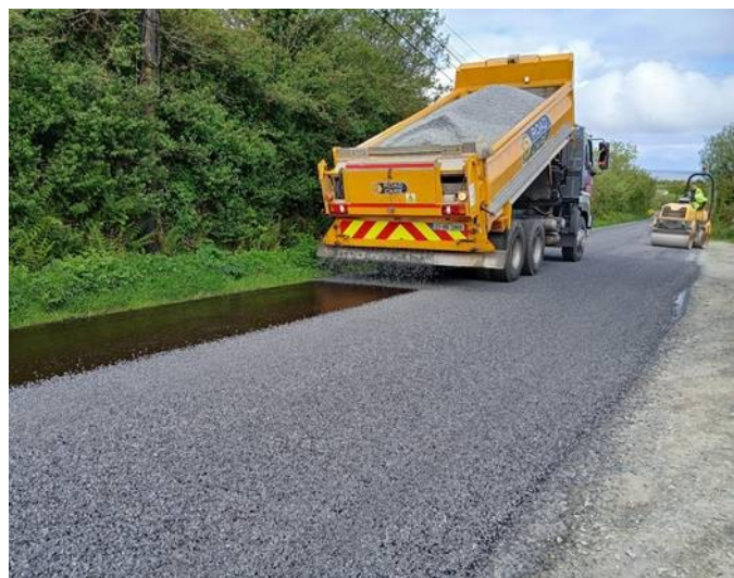
CN-RM-02 RENVYLE – 1.8KM SURFACE DRESSING BY DIRECT LABOUR STAFF IN CONAMARA NORTH
