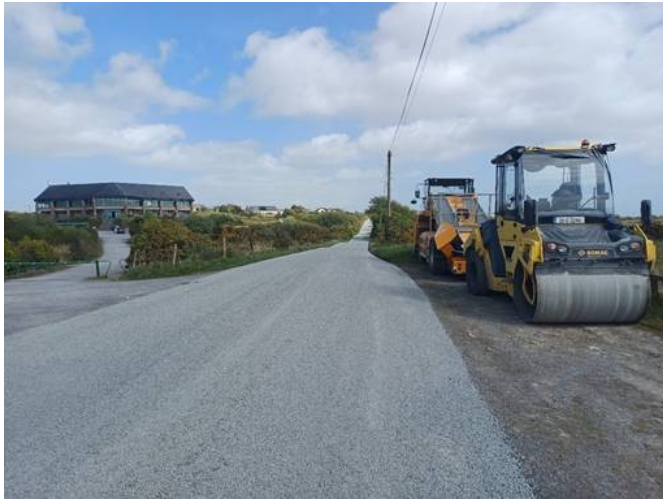
COLAS CONTRACTING HAVE STARTED ON THE CONAMARA SOUTH SURFACE DRESSING PROGRAMME. PHOTO TAKEN ON CS-RM-07 NEAR BEARNA GOLF CLUB, A 2KM LONG STRETCH
