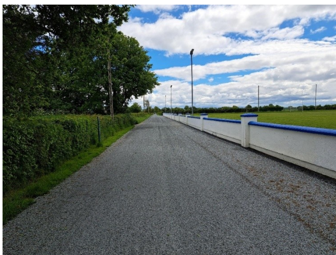
FINISHED SURFACE DRESSING ON TOP OF THE OVERLAY OF THE L-8726 AT BALLINAKILL, EYRECOURT.
