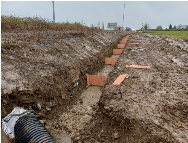
RECONSTRUCTION OF DAMAGED RETAINING WALL ALONG THE R446 AT AUGHRIM, FOUNDATION WORKS
