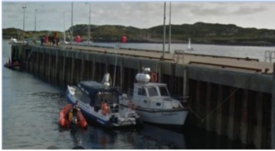
INISHBOFIN – RUBBER D-WING FENDERS & SLIPWAY BARRIER
