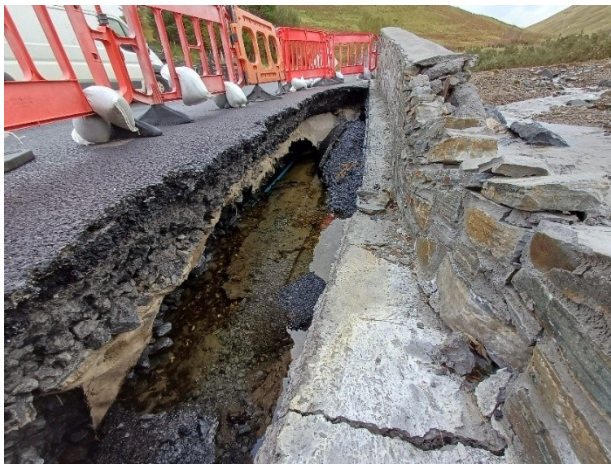
PHOTO WHICH SHOWS THE EXTENT OF THE UNDERMINING OF THE ROAD STRUCTURE - NA GRINGEACHA
