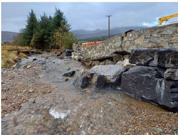
VIEW FROM THE RIVER OF THE DAMAGED ROCK ARMOUR - NA GRINGEACHA
