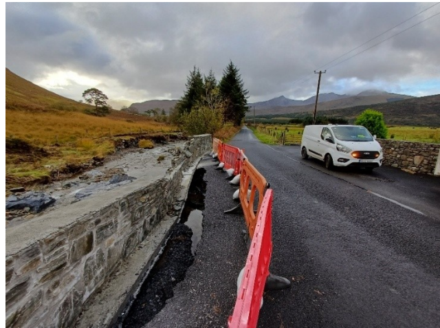
VIEW FROM THE ROAD SHOWING THE DAMAGE CAUSED TO THE ROAD STRUCTURE AND PARAPET WALL
