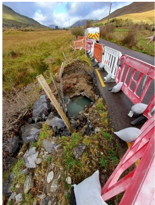
DAMAGE TO CULVERT AND ROAD EDGE - R336, MUINTIR EOGHAIN AREA
