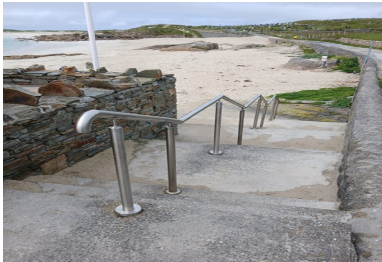
RECENTLY REPAIRED HANDRAIL TO GURTEEN BEACH ROUNDSTONE
