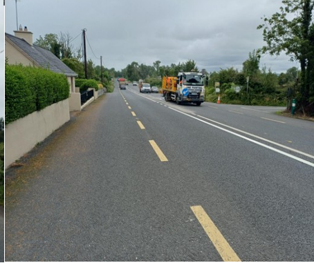
LOW-COST SAFETY IMPROVEMENT SCHEME ON THE R446 ON APPROACH TO CRAUGHWELL VILLAGE
