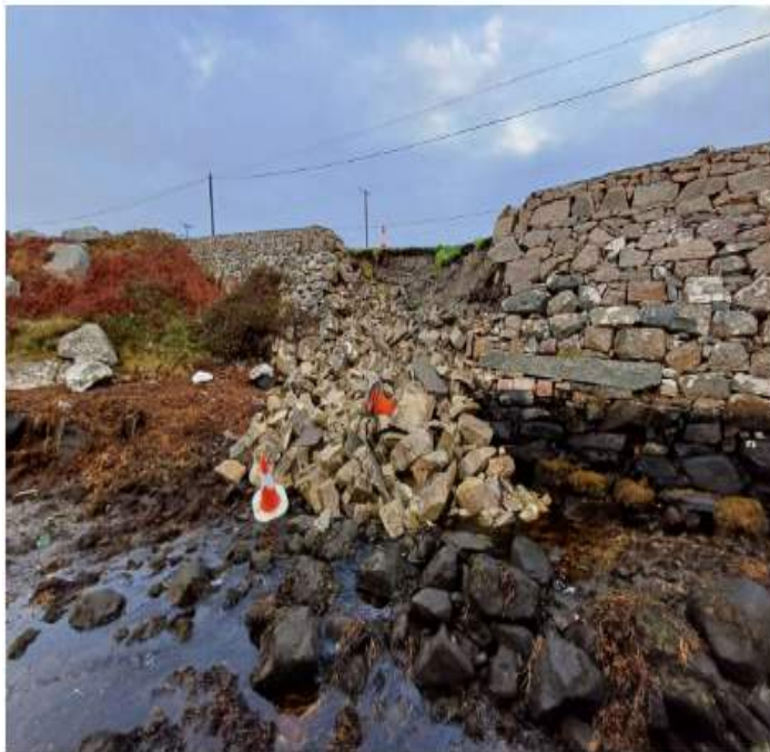
ROAD EMBANKMENT FAILURE, CNOC, LEITIR MEALLAIN
