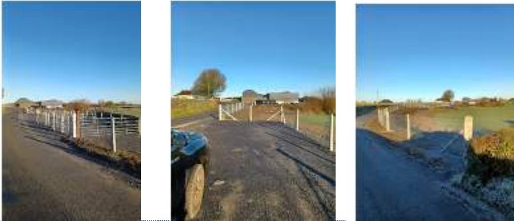
Community Involvement Scheme outside Headford which involved setting back boundary to improve sightlines for motorists and passing bays.
