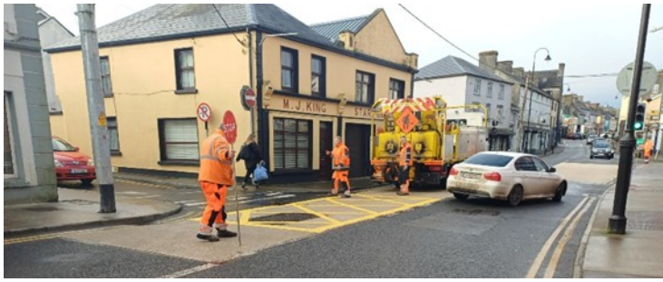
REINSTATING YELLOW BOX AT THE JUNCTION OF BRIDE STREET AND MOORE STREET, LOUGHREA.
