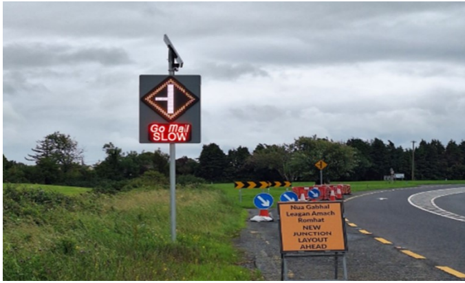
DERRYDONNELL ACTUATED SIGN
