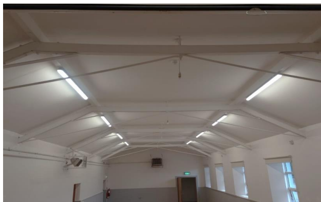
New Energy Efficiency Lighting at St Catherine's Hall in Aughrim
