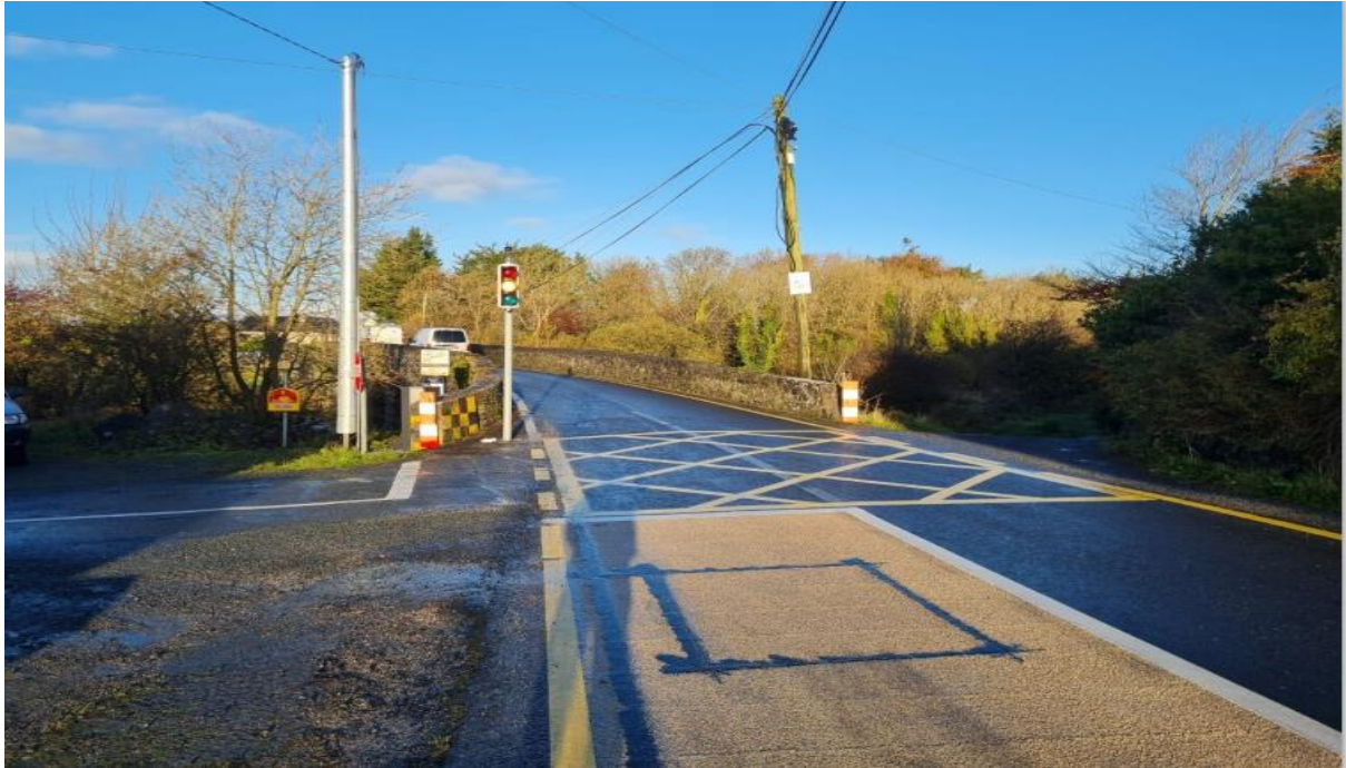
CREGMORE BRIDGE LIGHTS
